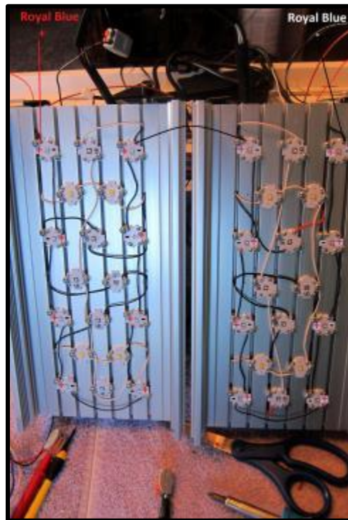
Figure 74: Wiring Completed with Royal Blue Circuit Highlighted
