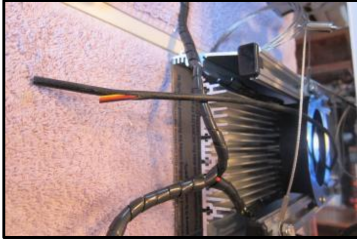
Figure 97: Fan with Molex Connectors Removed
