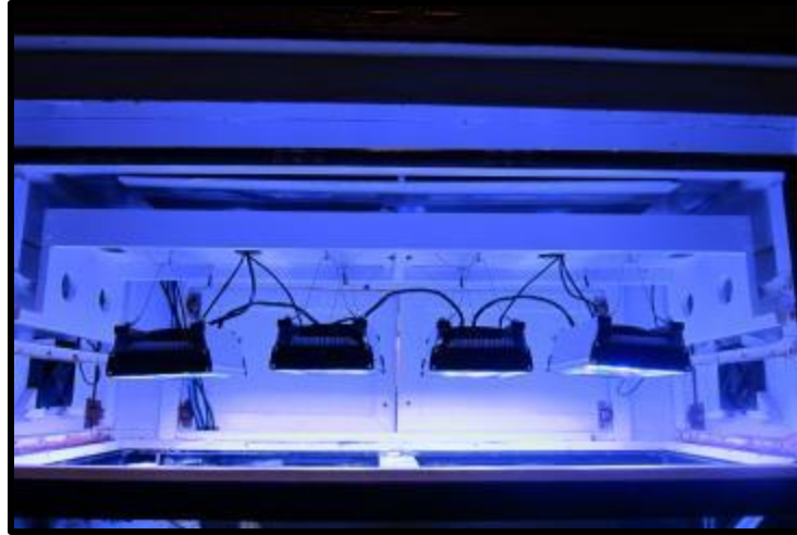
Figure 116: LED Light System Installed and Functioning
