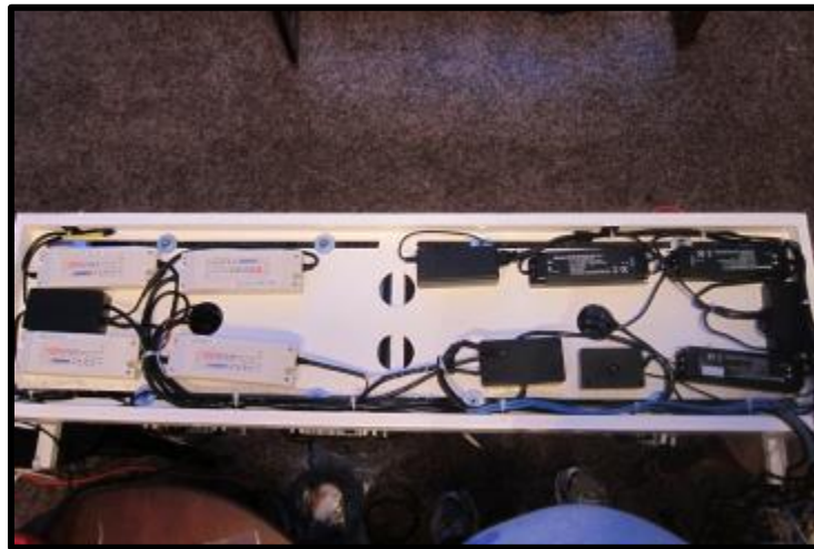
Figure 107: LED Light System Complete
